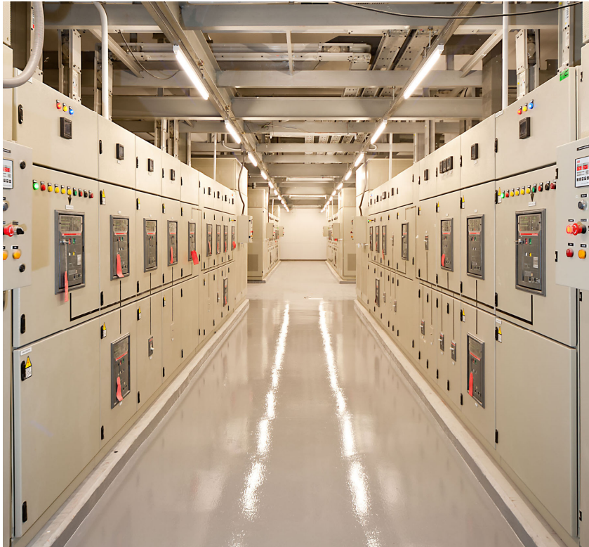
Modern low voltage industrial switchboard and motor control centre
