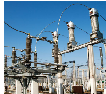
Outdoor high voltage substation
